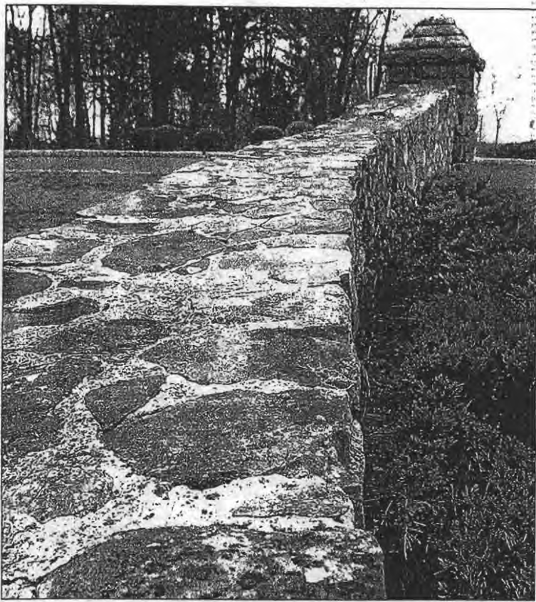
The stone wall in front of Montebello Park, along Hemion Road in Suffern, was recently restored.
